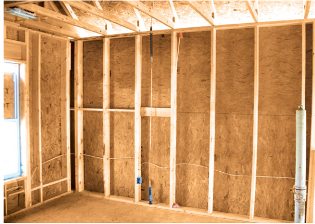
2x horizontal blocking between studs can be oriented with either the edge against the sheathing/drywall or the wide face vertical against the sheathing. Both options are shown.
