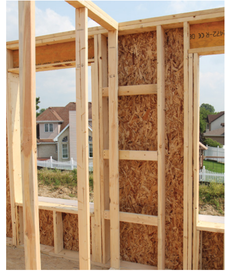
Ladder junctions at interior-exterior wall intersections (Figure 5) produce wall cavities that can be easily insulated to help builders earn the ENERGY STAR® label for new homes.
