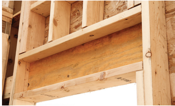
Advanced framing headers, such as single-ply headers, offer increased energy efficiency by replacing framing materials with space for cavity insulation inside the header (see Figure 7).
